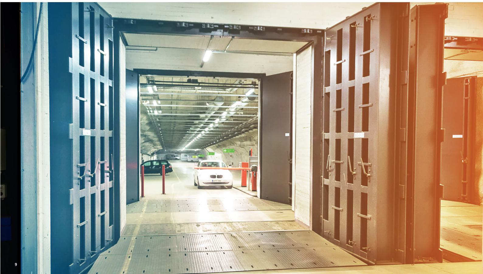
Double Leaf Blast Doors at the entrance of an underground car park
