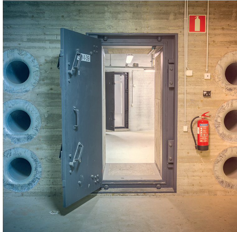
Blast Door and Blast Valves
